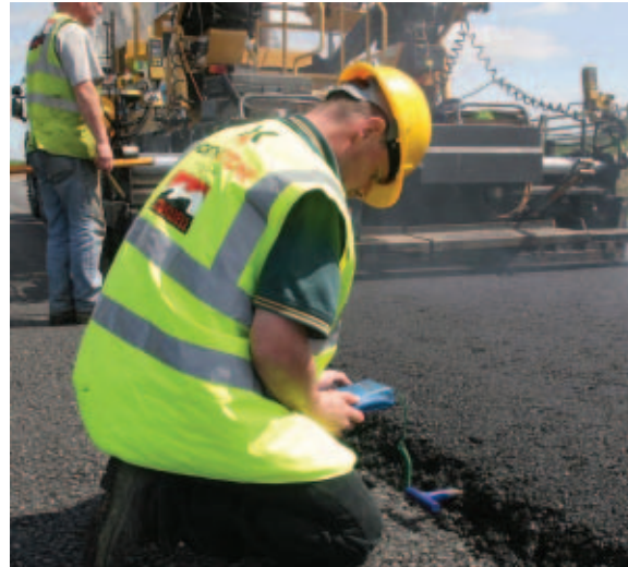
Taking Quality Seriously – Martin Kane checks product temperature on the newly laid surface at Bundoran
