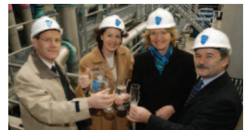
Left to right: Eamonn Sweeney toasts the official opening of Loughmacrory with Katharine Bryan (Chief Executive, Water Service), Libby Gawith (Earth Tech) and Trevor Haslett (Water Service). Eamonn's chosen tipples was of course, cool clear water from Lough Macrory.
