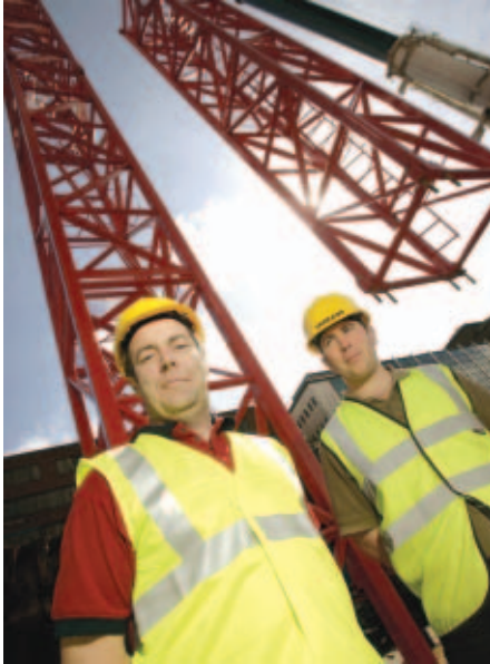
John McReynolds (left) and Shane Daly (right) oversee the mast erection on the first tower crane at Victoria Square
